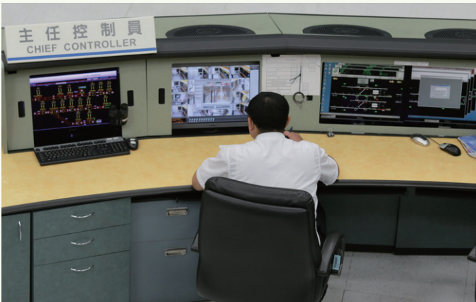
► Chief Controller is monitoring the entire station through computer screens.
